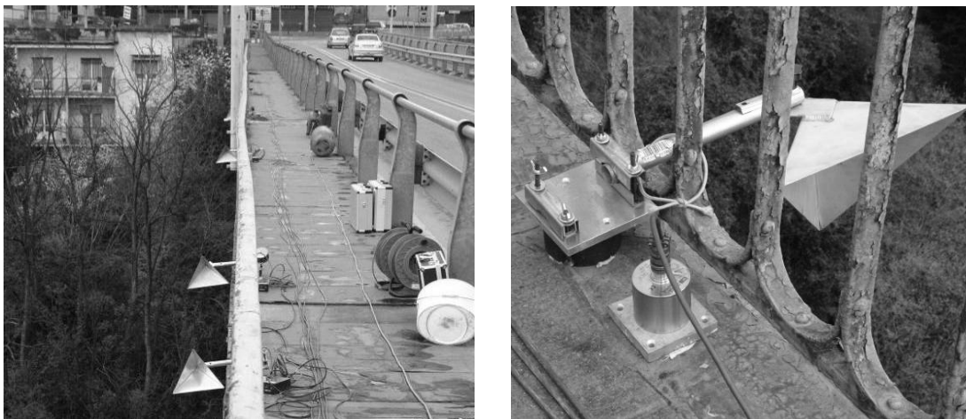
Figure 6: Accelerometers and corner reflectors installed on the Capriate bridge
