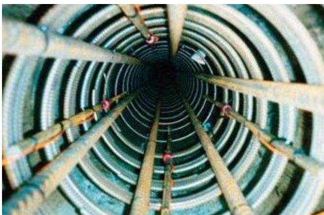
Four Sisters Bars are installed in the cage of a cast pile
