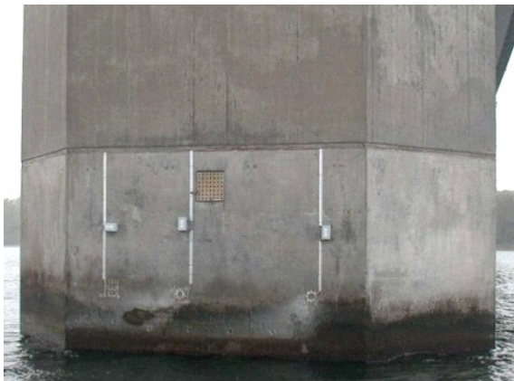
Figure 1. CorroRisk probes mounted on bridge pillar
